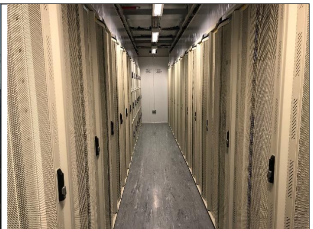
DATA HALL CUSTOMER RACKS
